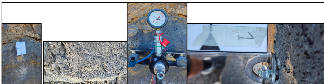
Figure 4 (a–d). Overview of test site 1, showing the black basalt rock type, the 6 kN pull-out test setup, and the observed movement at test (in column D) under an 8 kN load.
